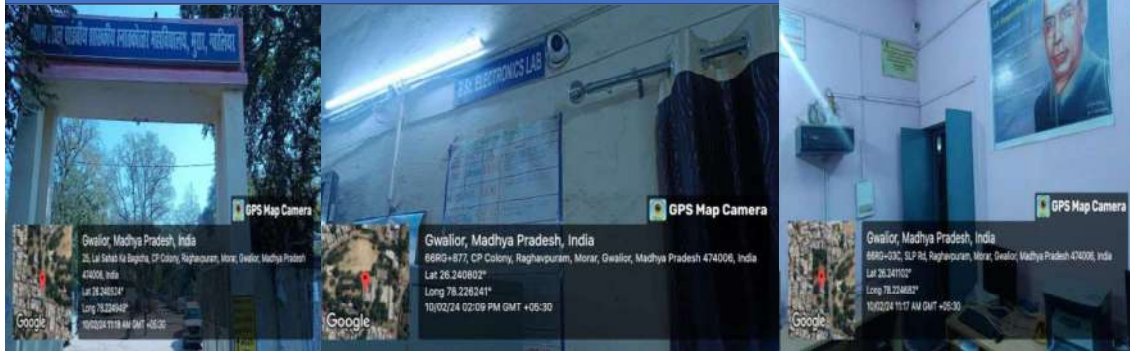
Photo 5: CCTV cameras on campus
